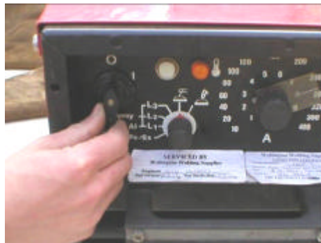
Figure 16: Switch Off the Welding Generator
