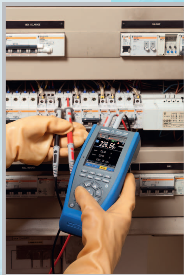
Measurements on electrical cabinets
