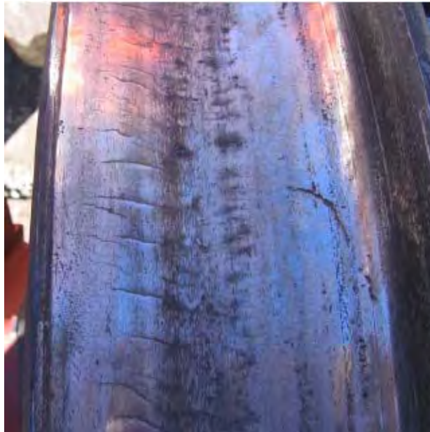
Photograph 6 Class 4 Rolling contact fatigue
