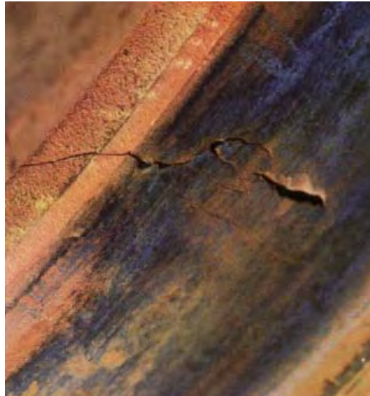
Photograph 11 Class 5 Fatigue Crack (propagated from a thermal crack)
