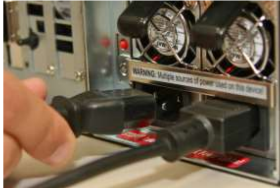
Figure 10: Power Cables Connected to ShowVault
