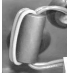
Figure 2-5: Ferrite core and battery supply wiring
