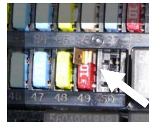
Bladed Fuse Power Tap Installed
