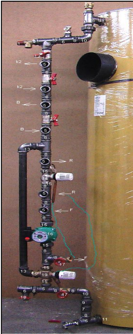
Fig. 4.1. Plumbing node. R - to/from radiator (s), F - to/from floor heating, B - to/from boiler, K2 - to/from other solid fuel boiler.
