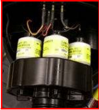
Installed Oxygen Sensors
