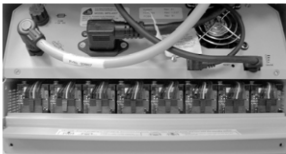
Properly seated connections
