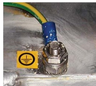
Place of connection of the earthing wire
