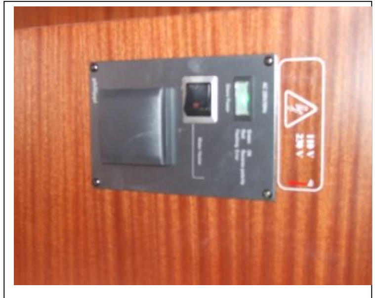
FIGURE 14: SHORE CONNECTION PANEL
