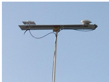
Figure 13 DKE Aerospace antenna mast with antennas
