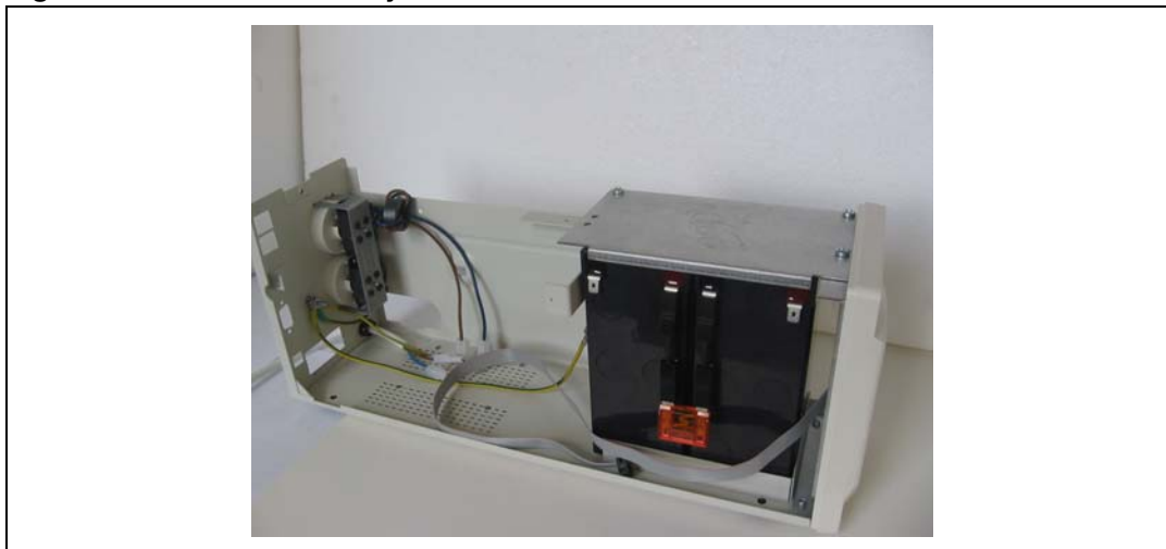
Figure 32. UPS with AVR transformer
