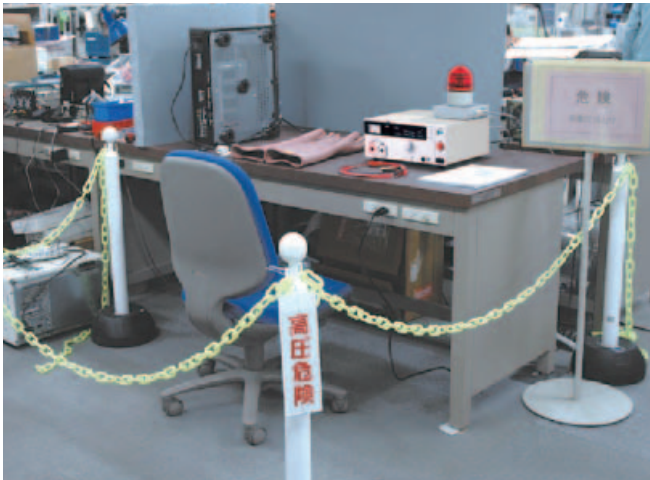
▲ The picture shown above indicates the caution sign of "HI VOLTAGE DANGER" with a chain surrounding the test site.
