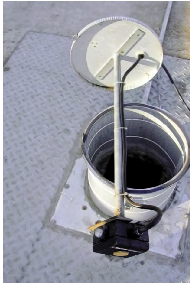
Picture 4: Smoke detector in a practical application
