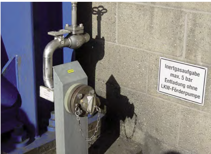
Picture 9: Inert gas connection to stationary evaporator
