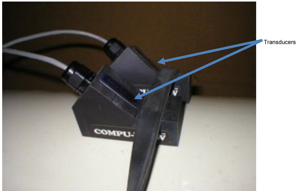
Figure 2-5. Clamp-on transducers secured with a bungee and chain
