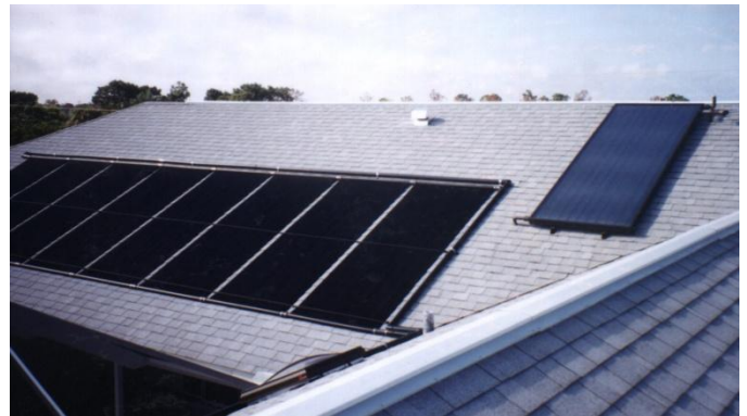
This photo shows two other non-PV solar collector types, a solar pool heater in the bottom left and a solar domestic hot water heater in the upper right. Although the solar water heater in the upper right may look similar to the PV modules in the grid tied example, the copper tubing extending off the upper right and bottom left of the collector indicates that these are hot water collectors. (Photo Credit – The Leveredge)
