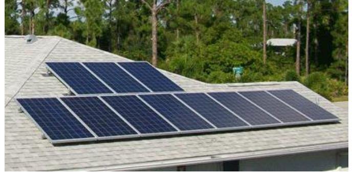
The example shown in the above photo is of a grid-tied solar electric (PV) system. PV module sizes vary and it is difficult to estimate the total system size in watts just by casual observation. This PV array consists of 11 PV modules rated at 230 watts STC each. (Photo Credit – Solar Power Electric™)
