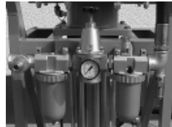
12 Air maintenance unit
