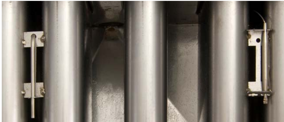
Typical sensor probe/high-limit locations and mounting hardware.
