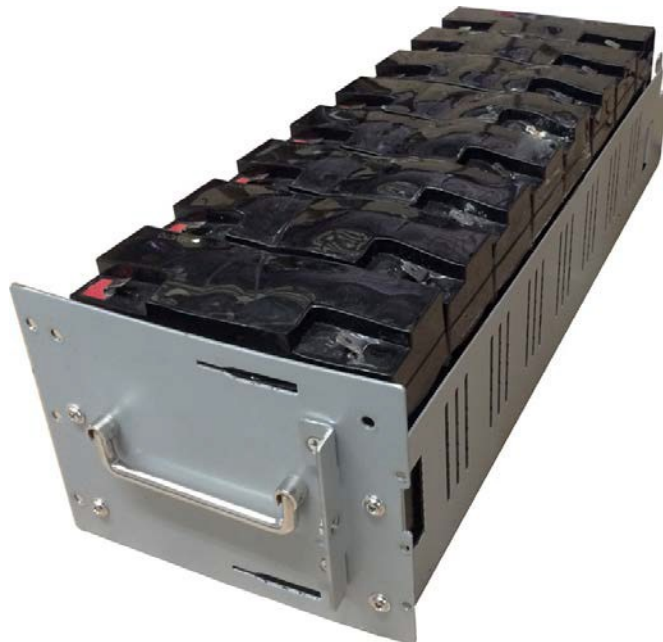
Example above of temperature affected batteries (shown without wires)
