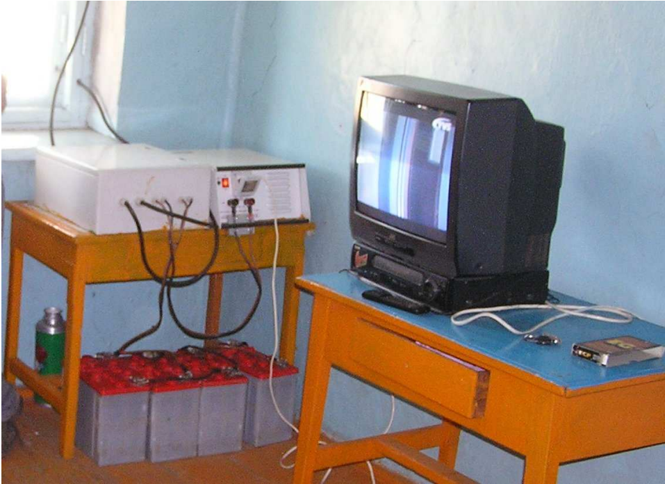
The regulator, inverter and batteries inside the school, giving electricity to a VHS and TV for teaching activity
