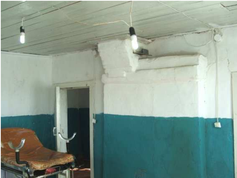
One of the rooms inside the hospital, with bulbs and switches provided by the project
