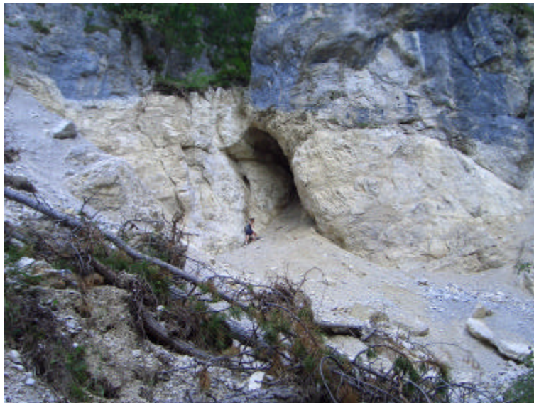
Fig. 5.2.1 - Erosion marks on a side slope of the Rio Cucco channel.
