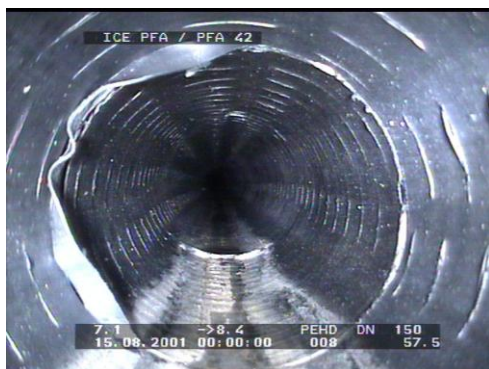
fig. 2.3.9 (1): drain pipe before repair
