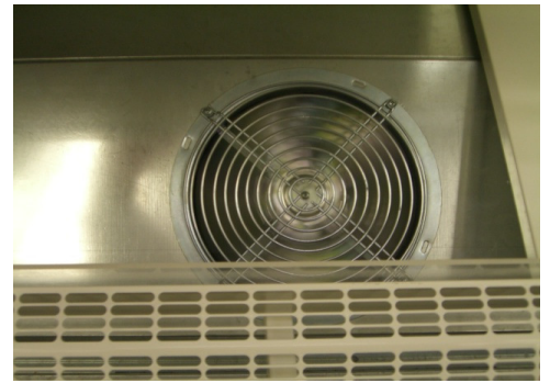
Clean around the fans
