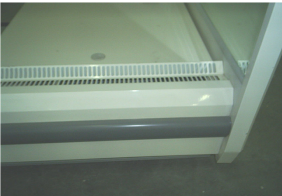
Make sure air return grille was open
