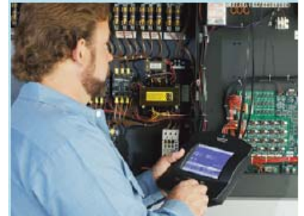
Monitors all key system functions and reports to alarm, if needed.
