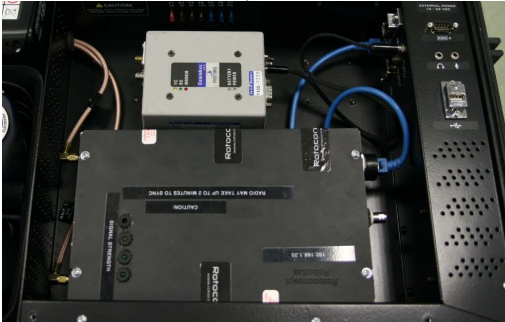
Figure 11 Example of hardware installation in MEC for an unmanned aircraft vehicle
