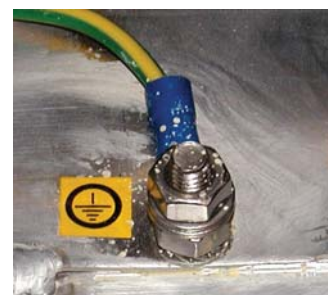
Place of connection of the earthing wire
