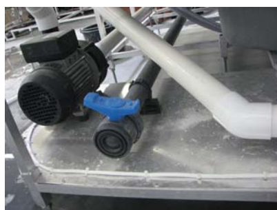
SPA Waterspace sewage outlet
