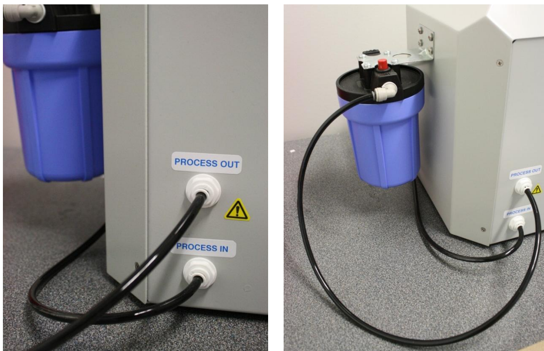
Figure 10. Coolant connections on the chiller
