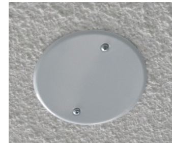
Ceiling Electrical Box
