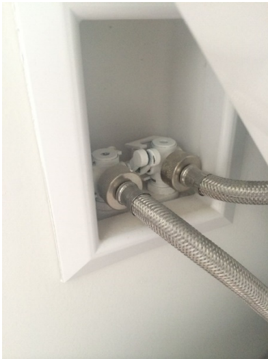
Water Shut-Off Valve
