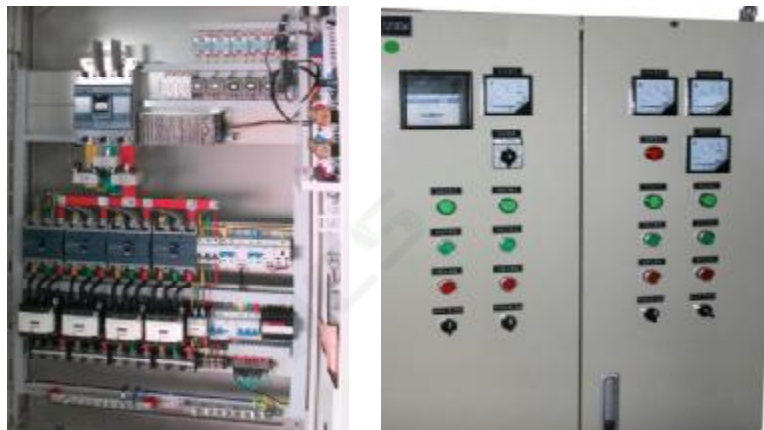
Image 3-20 Three-phase power cabinet
