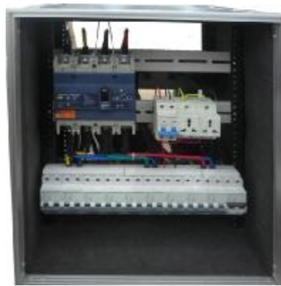
Image 3-19 Single-phase power box
