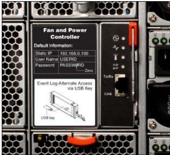
Figure 14. Fan and Power Controller
