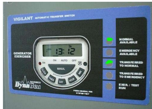
Incorrect LED alignment
