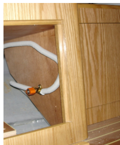
Gas supply valve under the stove
