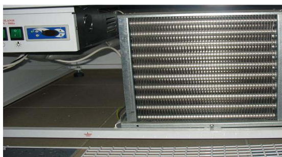
Fig.10 Cleaning the condenser
