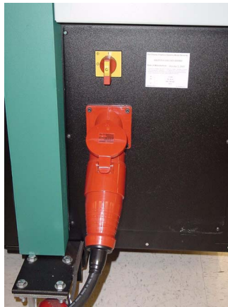
Figure 1-2 Circuit Breaker Switch Location
