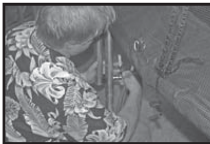
23- Secure all top mesh straps in tight bowties. Then, tighten all enclosure pole bolts and nuts. Finally, cover exposed threads with thread protectors.
