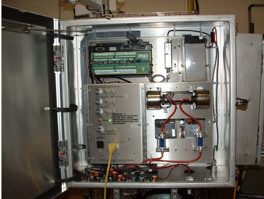
Figure 1-6 – Inside the FDCU
