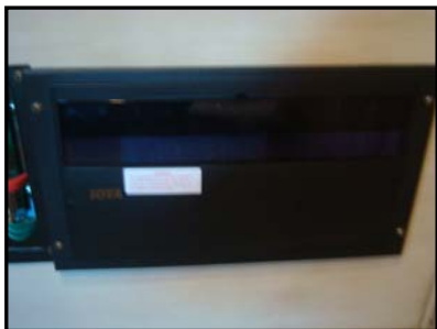
Figure 7-3. Circuit Breaker Box
