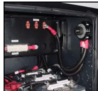
Figure 7-9. Rotary Switch to Disconnect “House” Batteries
