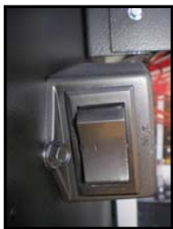
Figure 7-16. Power Switch for Generator
