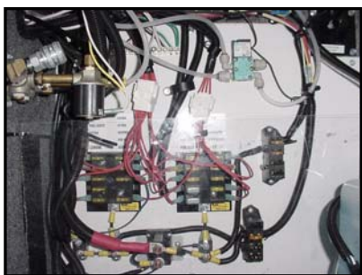
Figure 7-4. 12 VDC Fuse Panels
