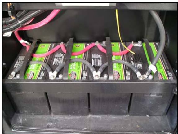
Figure 7-6. Maintenance Free House Batteries (Compartment)
