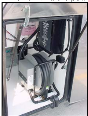
Figure 7-2. Electrical Power Hookup Cable
