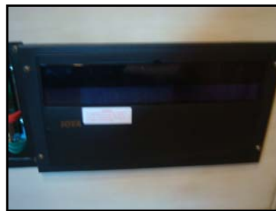
Figure 7-1. Circuit Breakers Located Under Refrigerator or in Bedroom Closet
