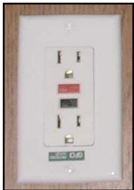
Figure 7-13. Ground-Fault Circuit Interrupter (GFCI)
