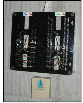
Wiring Center & Junction Box
