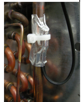
Thermistor attached to the refrigerant line.
