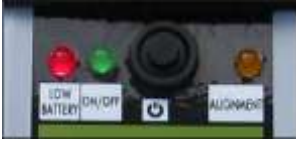
Fig. 15: Red LED lit indicates the batteries are low and need to be replaced. The system may not work properly with low batteries power.
