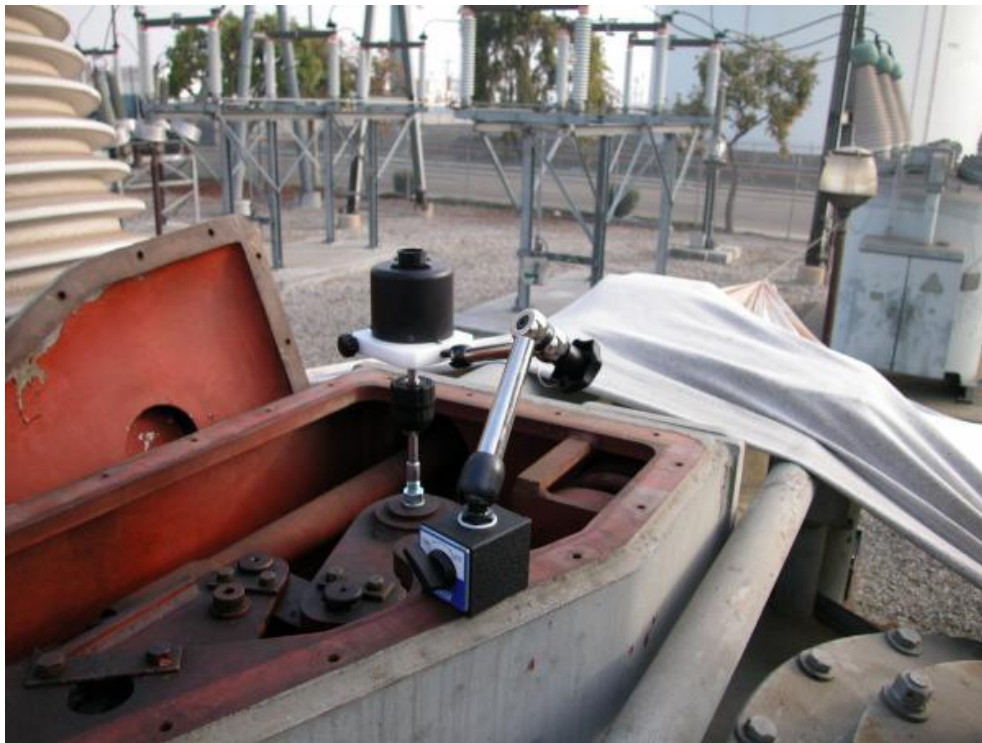
Rotary Transducer on Federal Pacific Circuit Breaker
