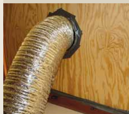
FIGURE 6 Flex duct connected to window template. The other end of the flex duct should be connected to the HEPA machine.
