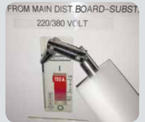
Ensuring no access with the jointed test finger on distribution board.
