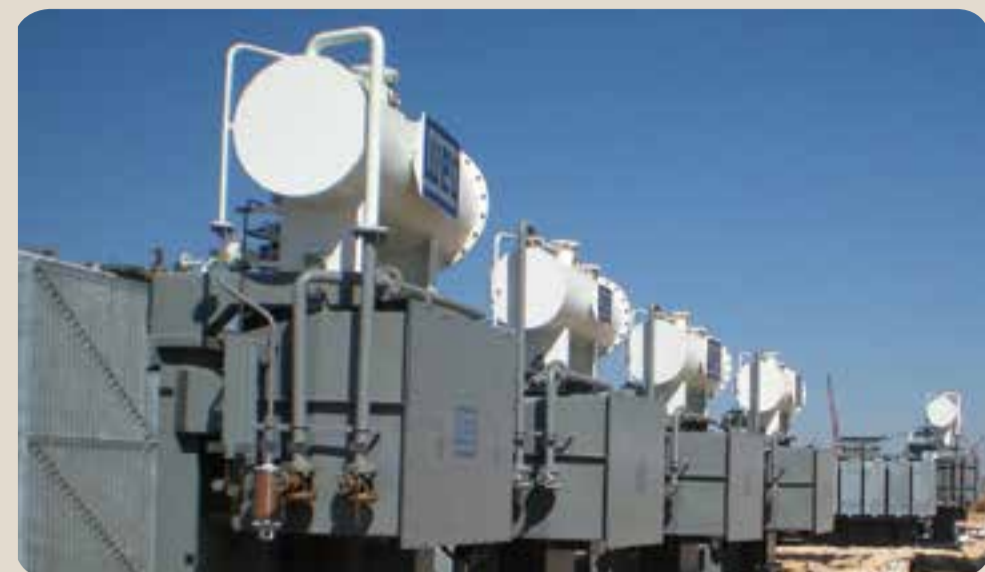
Four 7.5 MVA and one 20 MVA WEG transformers, part of the eighteen transformers delivered to Eskom's new Kusile coal-fired power station by Zest WEG Group.
