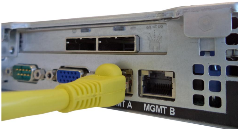
Rear Panel of the Bridge Showing Ethernet Cable Connections
