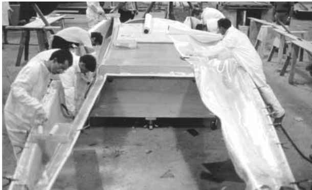
Figure 4-2 Fiberglass cloth is wet out in the bottom (hull) mold of the 32' catamaran after the cured epoxy gelcoat is washed and sanded.
