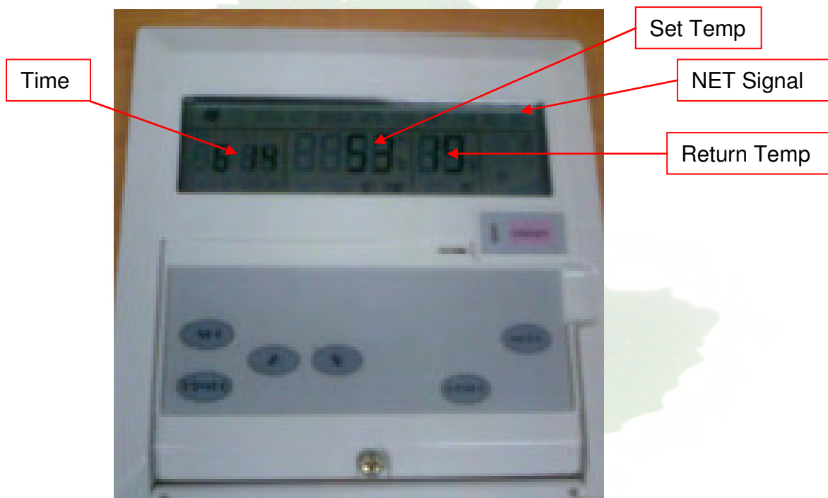
Figure 4: Heat Pumps control panel
