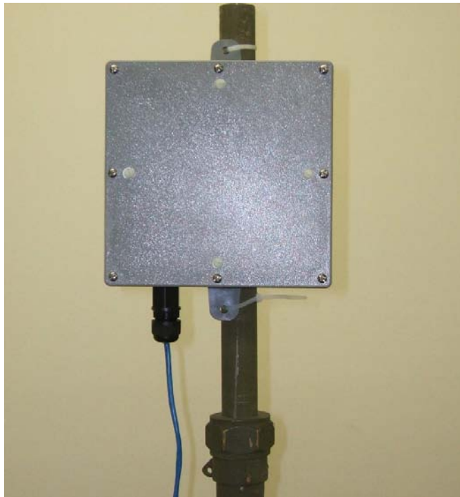
Figure 17: Pole Mounted Receiver Module Connected the DOG Base Station
