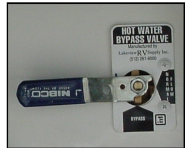
Figure 11-7. Water Heater Bypass Valve
