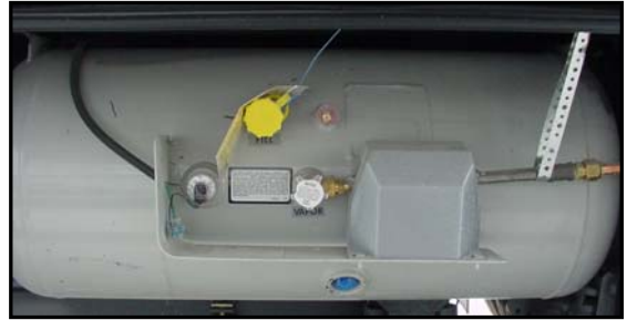
Figure 3-4. Liquid Propane Tank
