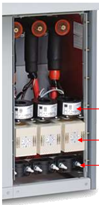
Current transformers for protection
